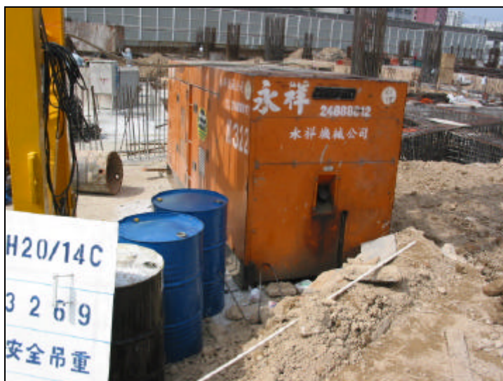
Figure 6-2 Generator and diesel drums without drip-tray
