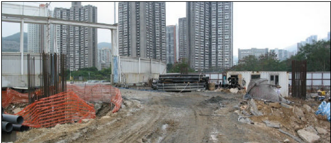
Figure 6-1 No wheel washing facility was provided at site access
