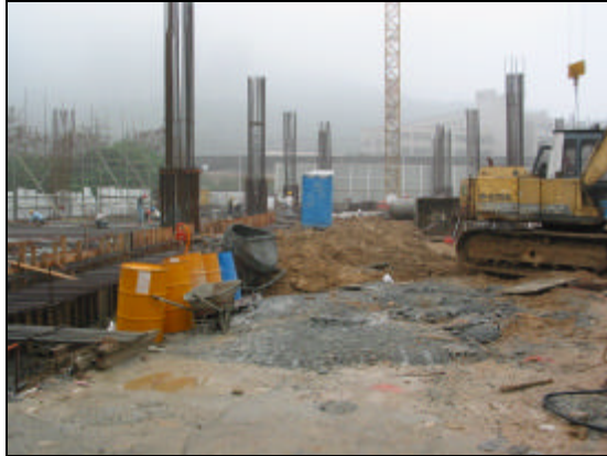
Figure 6-2 No drip-tray was provided for the diesel drums
