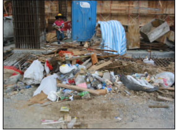
Figure 6-3 Rubbish at the site
