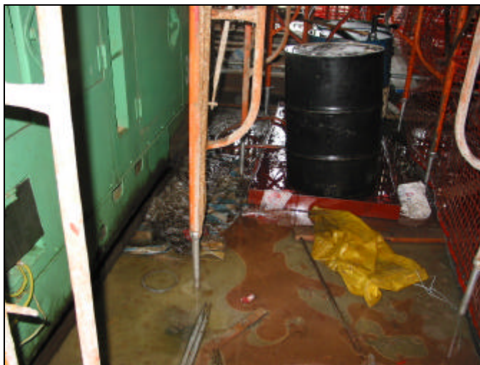
Figure 6-1 Oil spillage from drip tray
