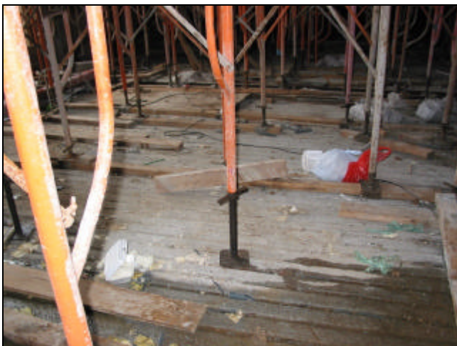
Figure 6-1 Rubbish at the 1/F of depot.
