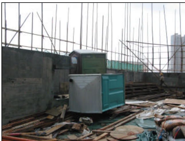
Figure 6-1 The collapsed chemical toilet on 3/F.
