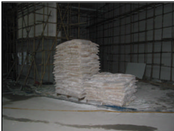
Figure 6-1 Cement bags without covering.
