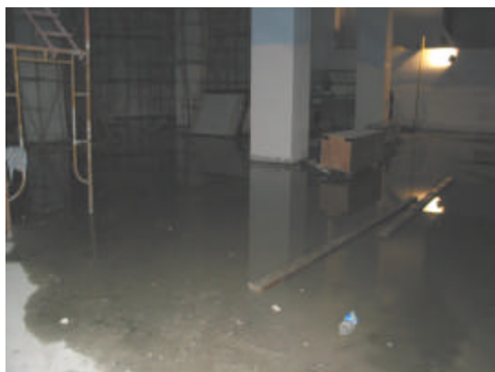
Figure 6-1 Stagnant water in Level 1
