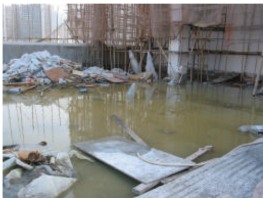
Figure 6-1 Stagnant water in Level 3
