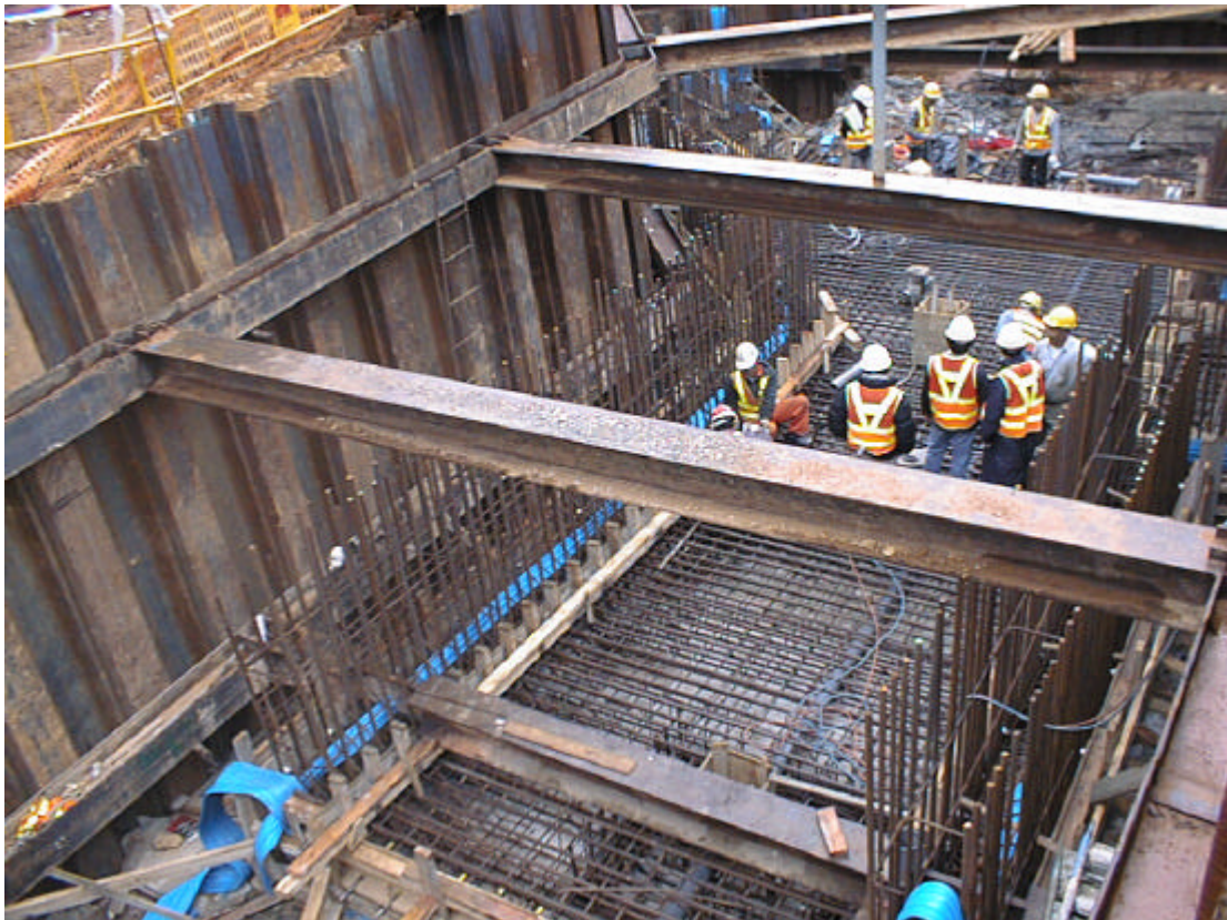
Date: 20 March 2003 Works: Construction of Subway Location: Sai Sha Road near Villa Athena
