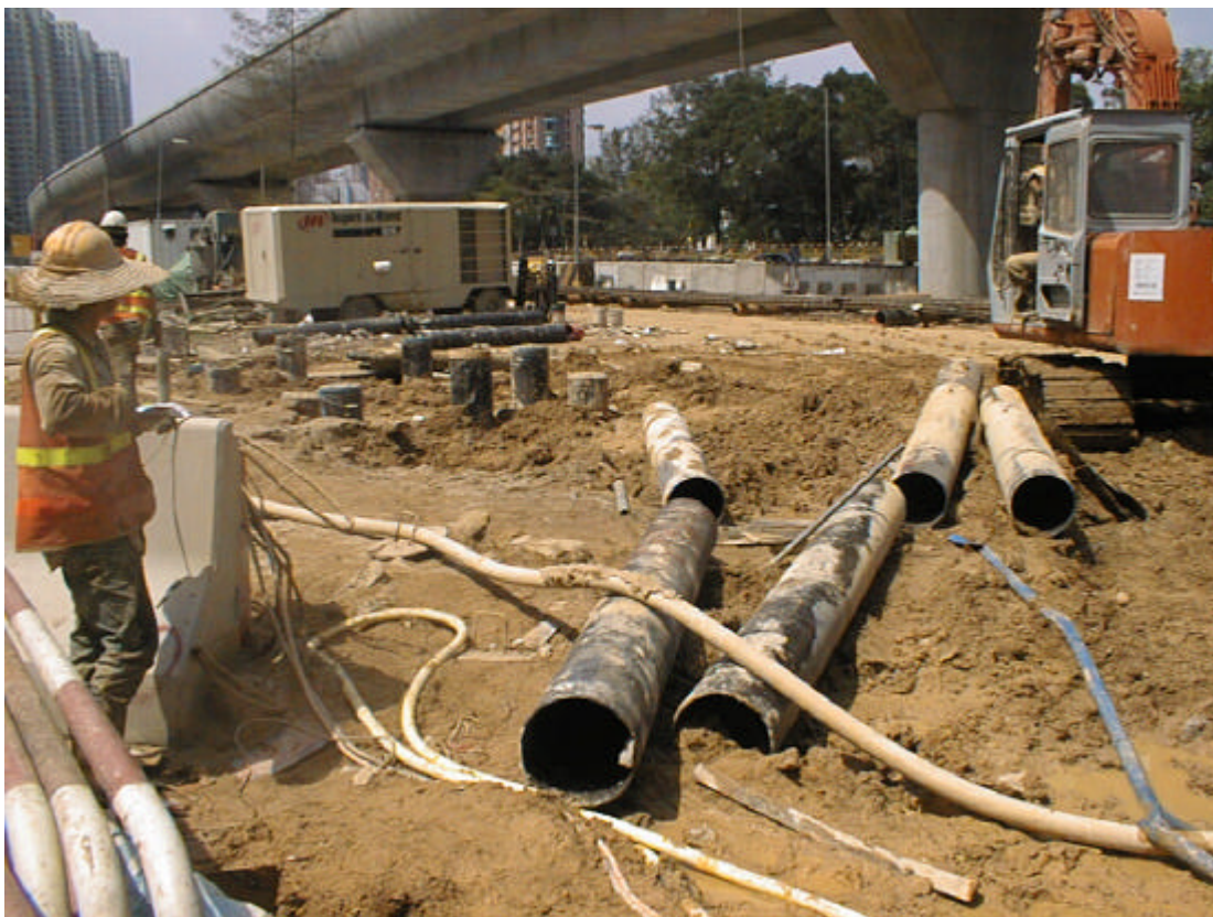
Date: 27 March 2003 Works: Construction of Footbridge Foundation Location: Sai Sha Road near Lee On Estate Lee Wing House
