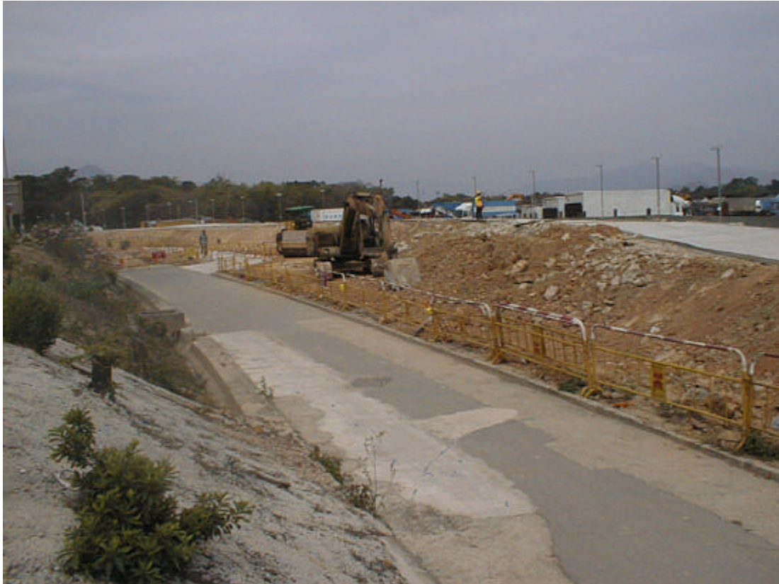
Date: 13 March 2003 Works: Construction of Temporary Access Road Location: Sai Sha Road near Residential Development at Wu Kai Sha DD 206
