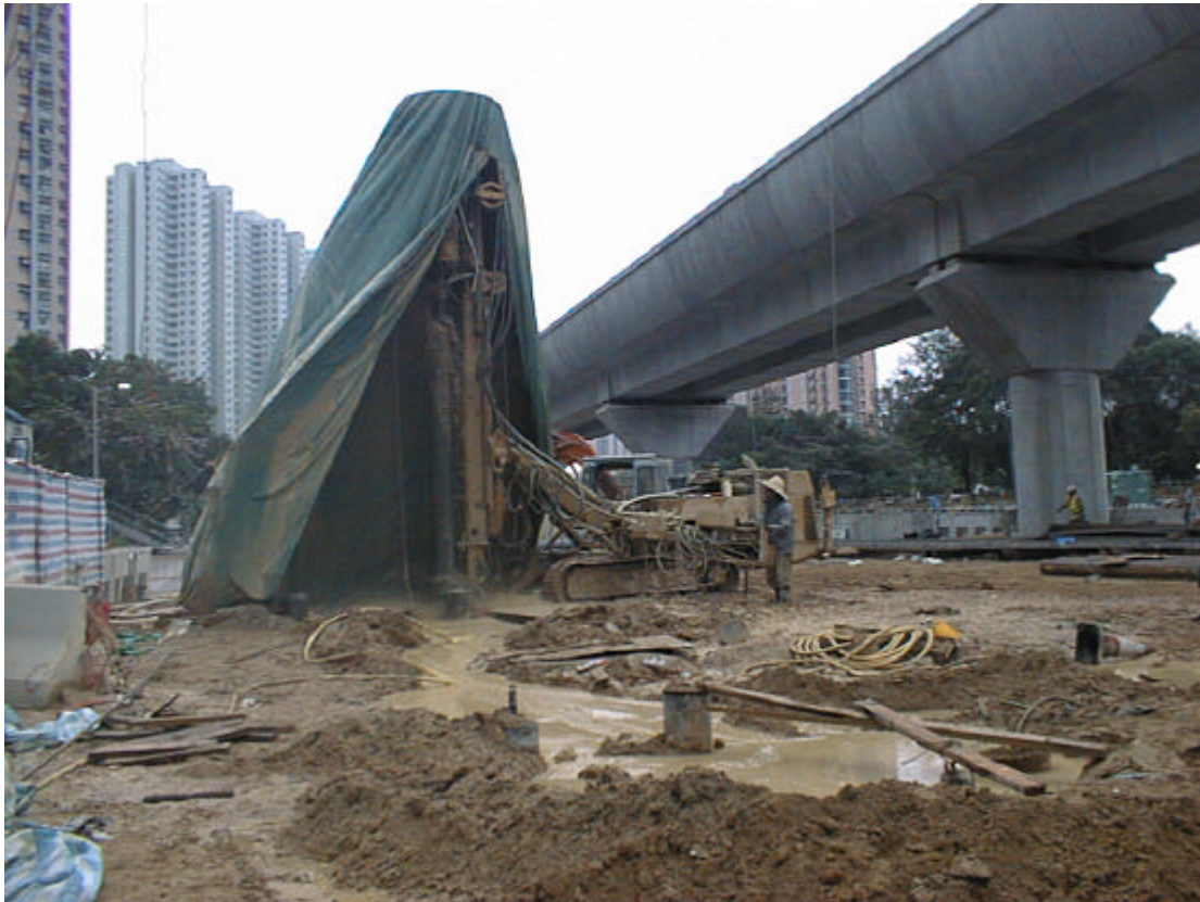
Date: 20 March 2003 Works: Construction of Footbridge Foundation Location: Sai Sha Road near Lee On Estate Lee Wing House
