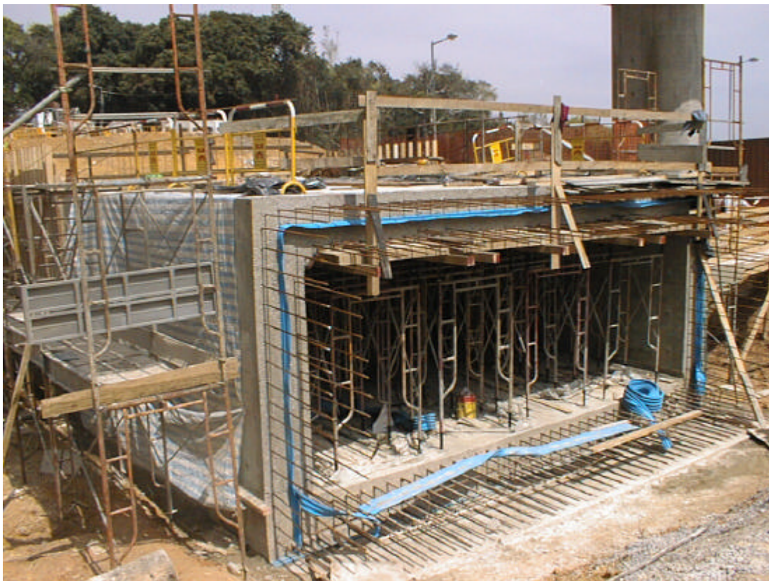
Date: 17 March 2003 Works: Construction of Subway Location: Sai Sha Road near Lee On Estate
