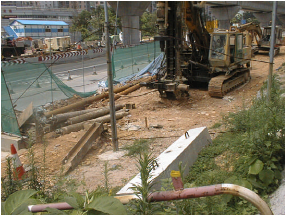
Date: 22 May 2003 Works: Mini pile works for Footbridge Location: Wu Kwai Sha New Village Access Road
