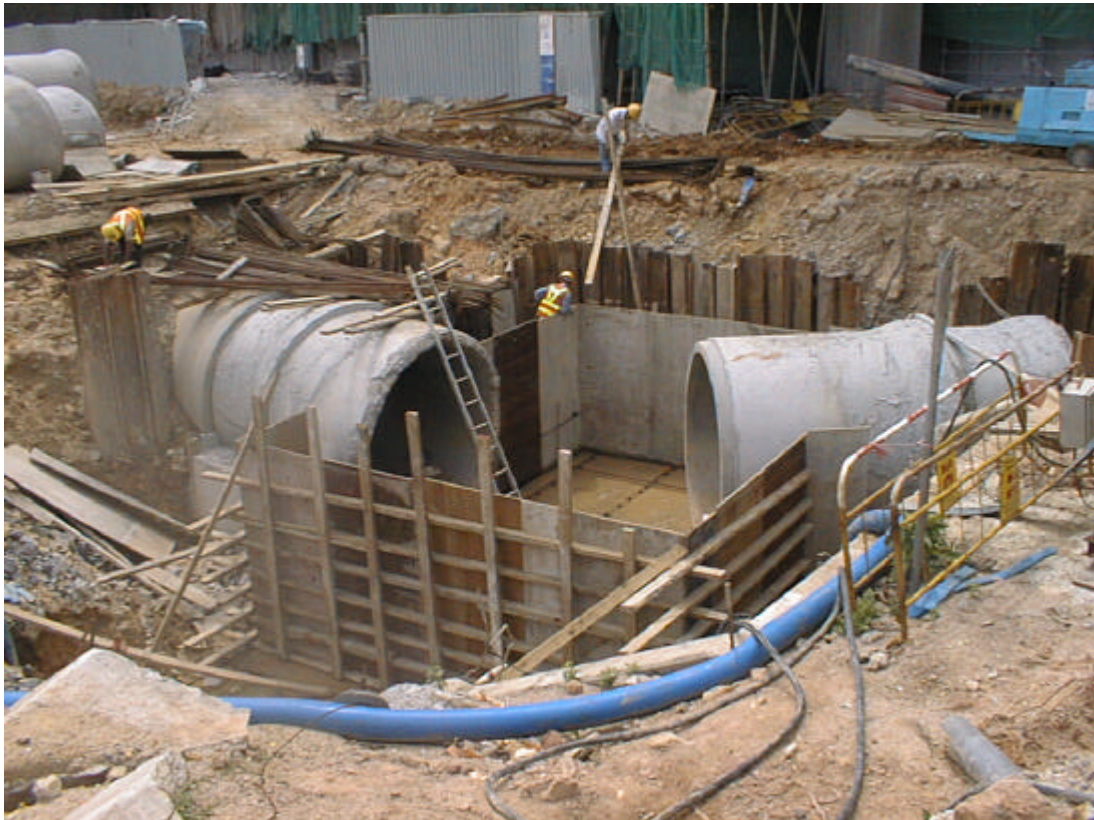
Date: 13 May 2003 Works: Construction of Manhole Location: Sai Sha Road near Wu Kai Sha Railway Station
