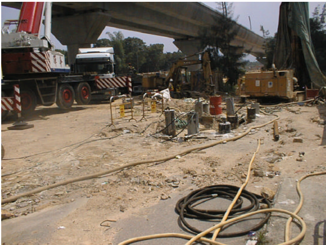
Date: 22 May 2003 Works: Mini pile works for Footbridge Location: Sai Sha Road near Lee Wing House
