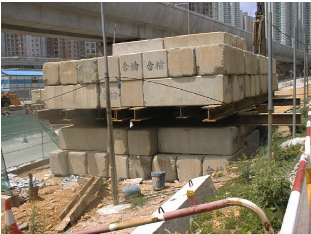
Date: 13 May 2003 Works: Loading Test for Footbridge Foundation Location: Wu Kwai Sha New Village Access Road
