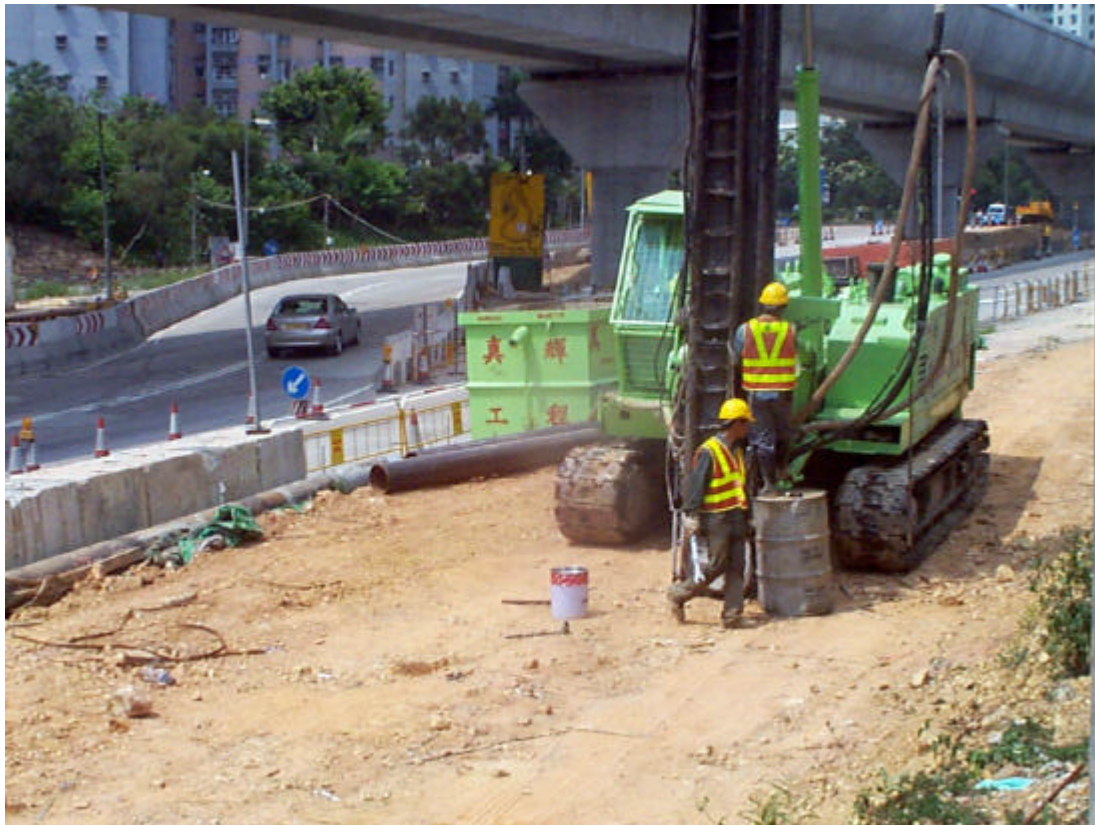
Date: 5 June 2003 Works: Minipile Works for Footbridge Location: Wu Kwai Sha New Village Access Road
