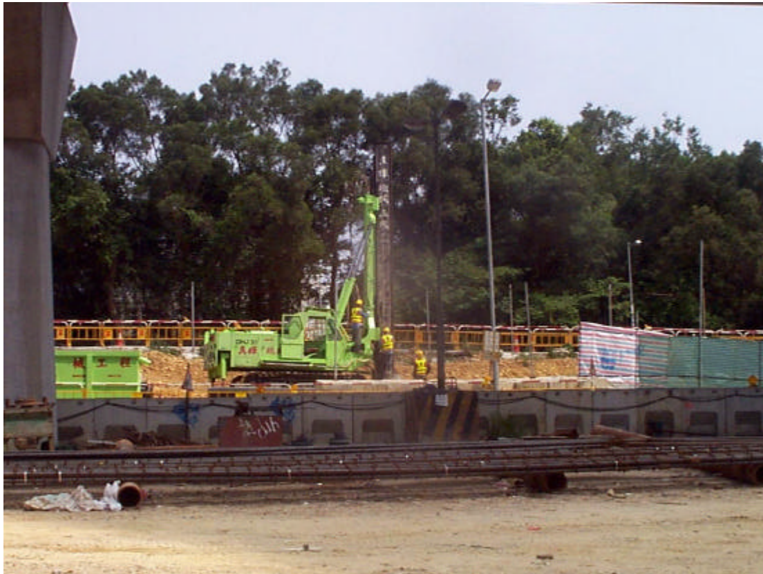
Date: 5 June 2003 Works: Minipile Works for Footbridge Location: Wu Kwai Sha New Village Access Road
