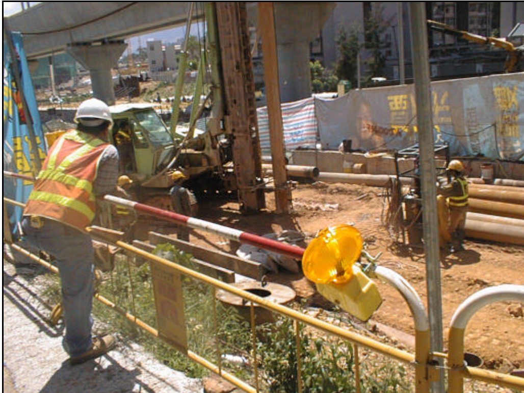
Date: 3 July 2003 Works: Minipile Works for Footbridge Location: Wu Kwai Sha New Village Access Road
