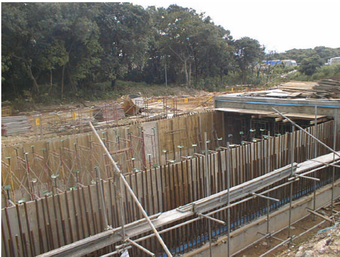
Date: 10 July 2003 Works: Construction of Subway Location: Near Residential Development Wu Kai Sha DD 206
