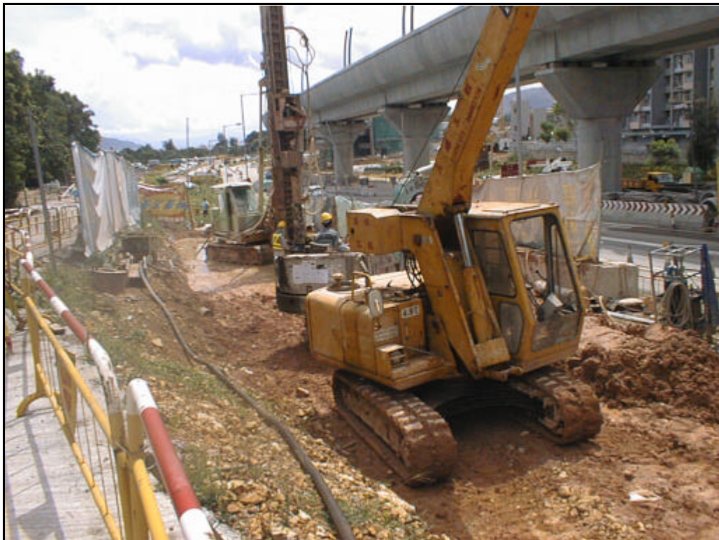
Date: 10 July 2003 Works: Minipile Works for Footbridge Location: Wu Kwai Sha New Village Access Road
