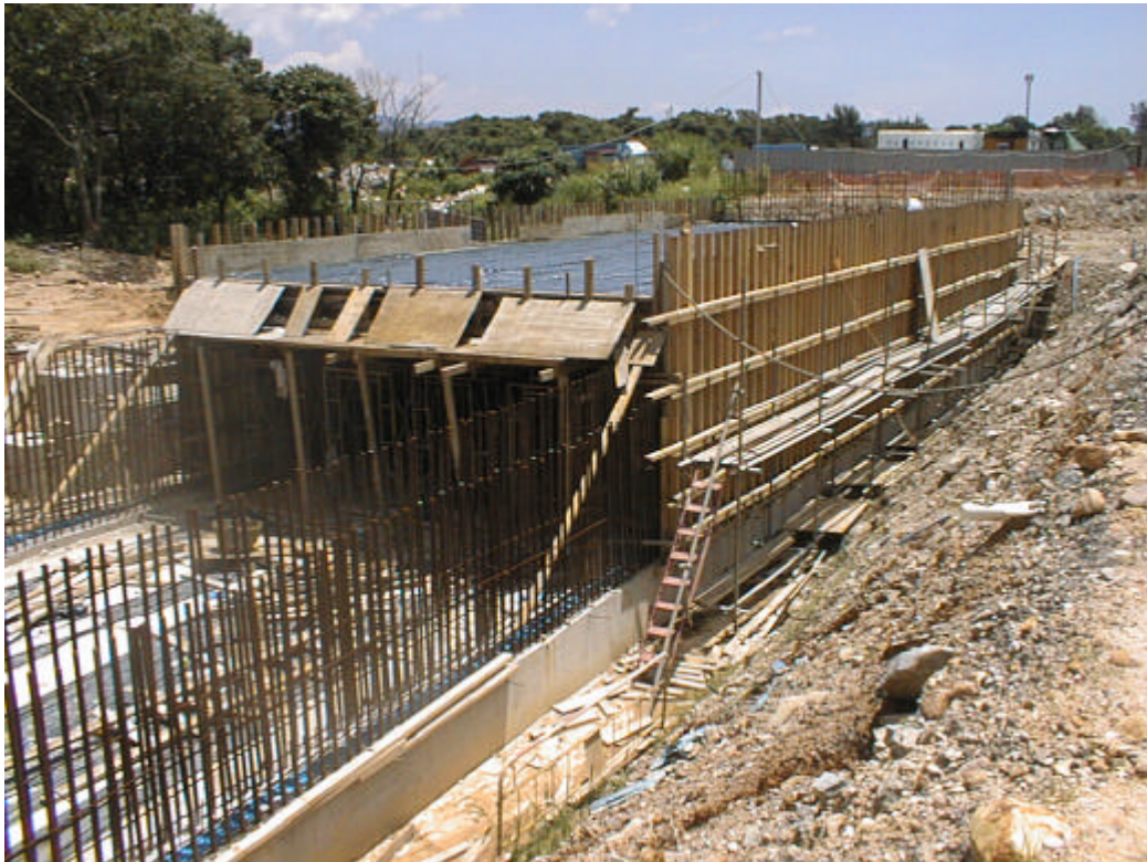
Date: 3 July 2003 Works: Construction of Subway Location: Near Residential Development Wu Kai Sha DD 206
