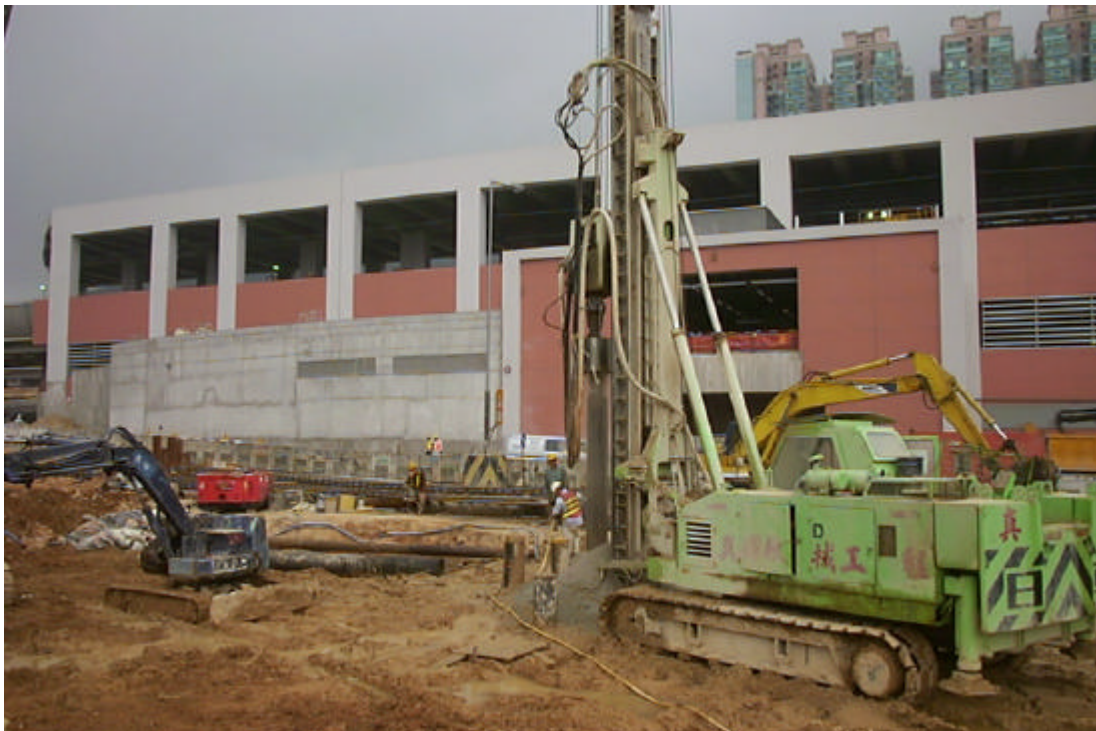
Date: 18 March 2004 Works: Mini-pile Construction Location: Near Residential Development at Wu Kai Sha DD 206
