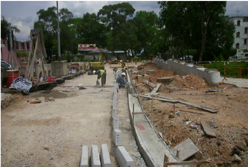
Date: 13 May 2004 Works: Road Work Location: Near Wu Kwai Sha New Village
