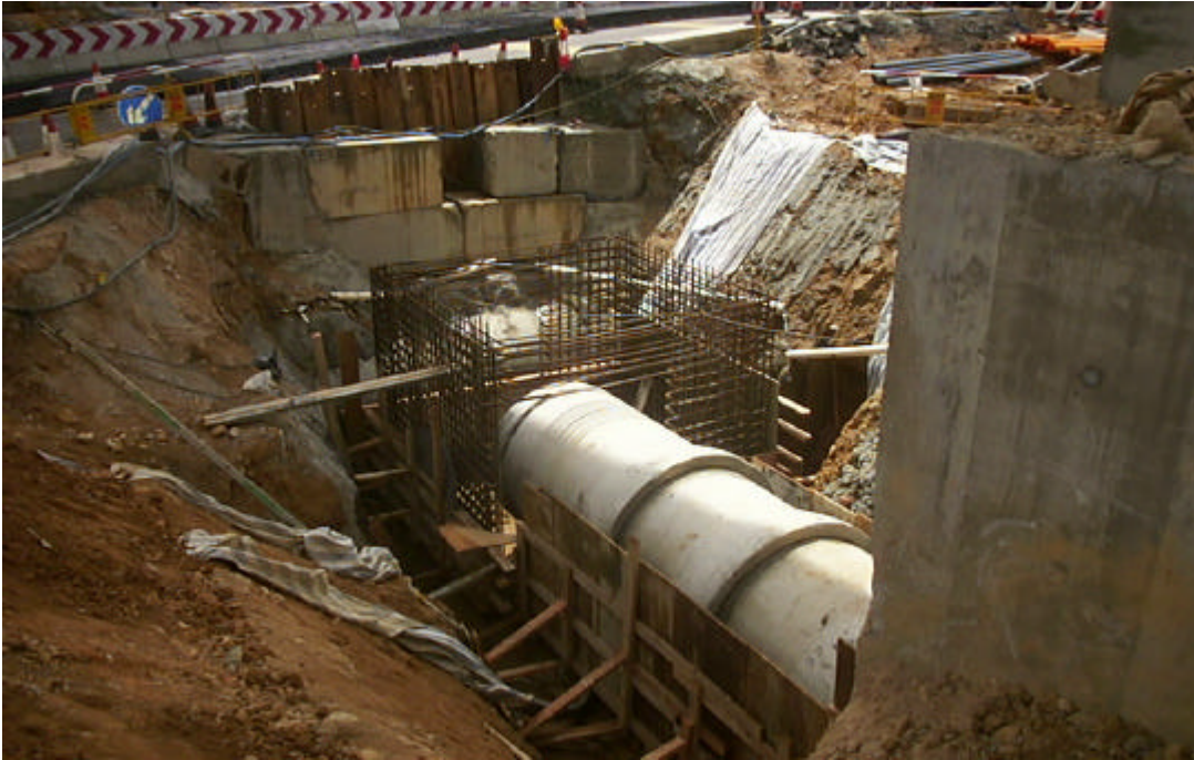
Date: 24 June 2004 Works: Drainage Works Location: Near Wu Kwai Sha KCRC Station
