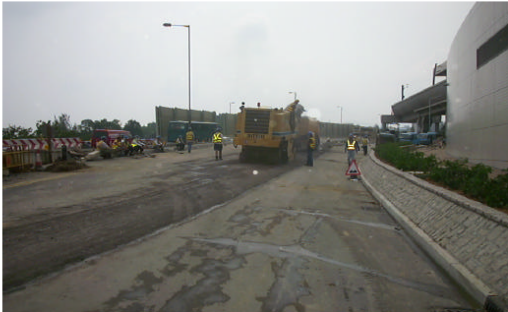
Date: 10 June 2004 Works: Road Work Location: Near Wu Kwai Sha KCRC Station
