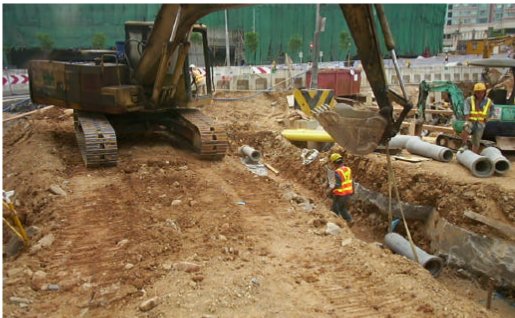
Date: 10 June 2004 Works: Drainage Work Location: Near Wu Kwai Sha KCRC Station
