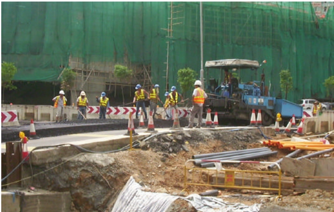
Date: 24 June 2004 Works: Road Work Location: Near Wu Kwai Sha KCRC Station
