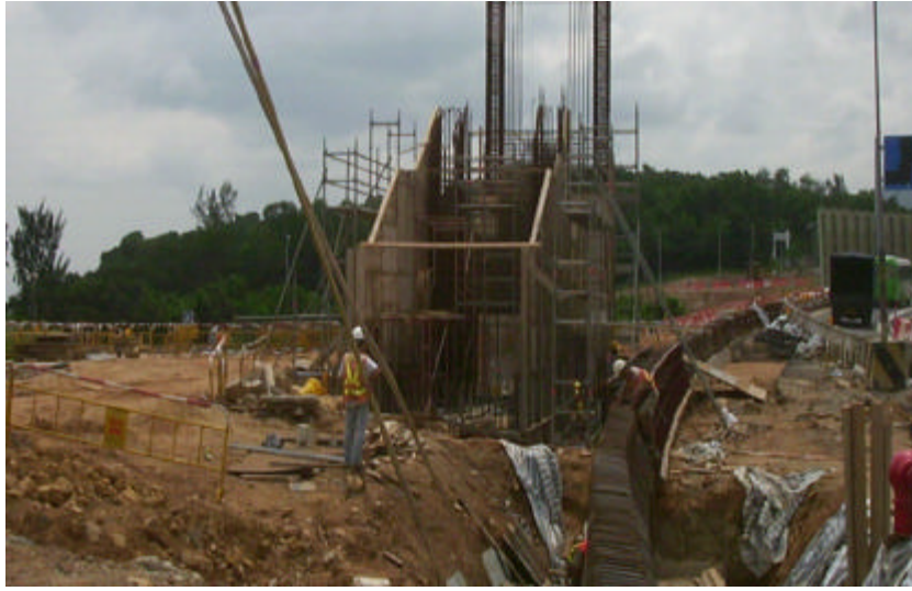
Date: 8 July 2004 Works: Staircase Construction Location: Near Residential Development at Wu Kai Sha DD 206
