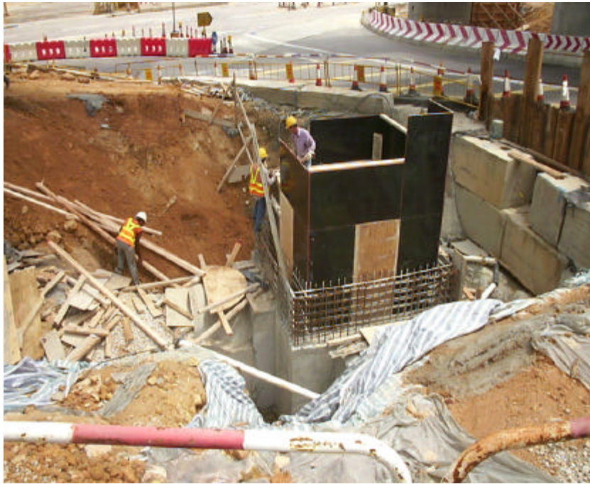
Date: 8 July 2004 Works: Drainage Work Location: Near Wu Kwai Sha KCRC Station
