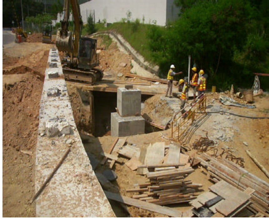
Date: 2 July 2004 Works: Drainage Works Location: Near Wu Kwai Sha KCRC Station
