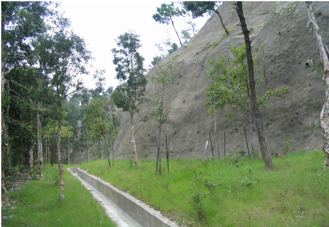
Plate No. 6 Newly planted trees and hydroseeded area along the slope toe
