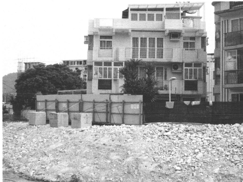
Photo 2: Erection of hoarding along the boundary of the site near House No. 105.
