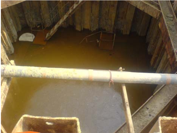
The Contractor was reminded to spray larvicide on persistent stagnant water to prevent breeding of mosquito.
