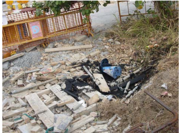
Lube oil splashes was observed at Nam San Wai Road site near King Fai Farm, the Contractor was reminded to remove the timber and the stained soil as chemical waste.
