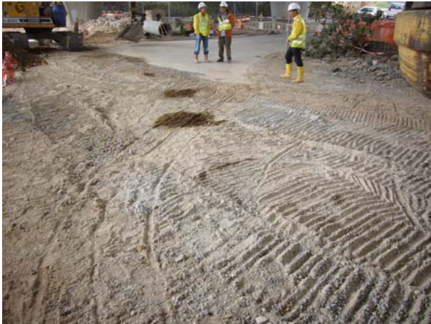
Oil stain patch was observed at Nam San Wai Road Portion H, the Contractor was reminded to clean and the removed soil should transfer to chemical waste storage area.
