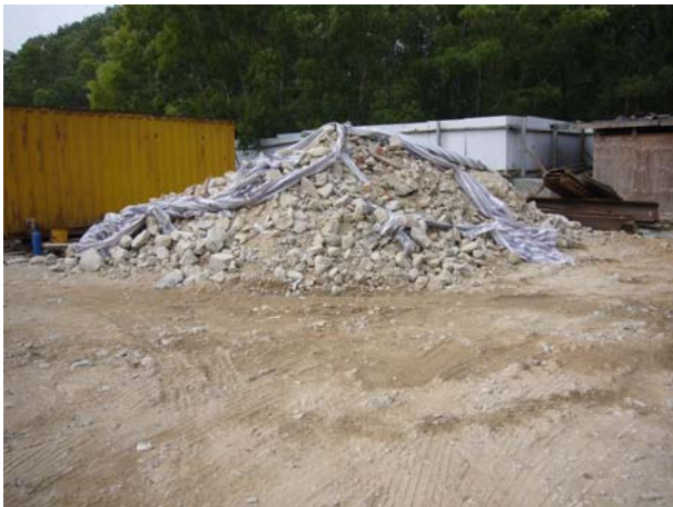
Stockpile without cover was observed, the contractor was reminded to cover properly to prevent dust generation.
