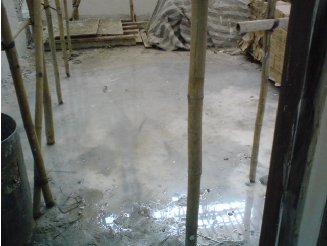
Stagnant water was accumulated inside the pumping station at Nam Sang Wai Station, The Contractor was remained to drain away the stagnant water.
