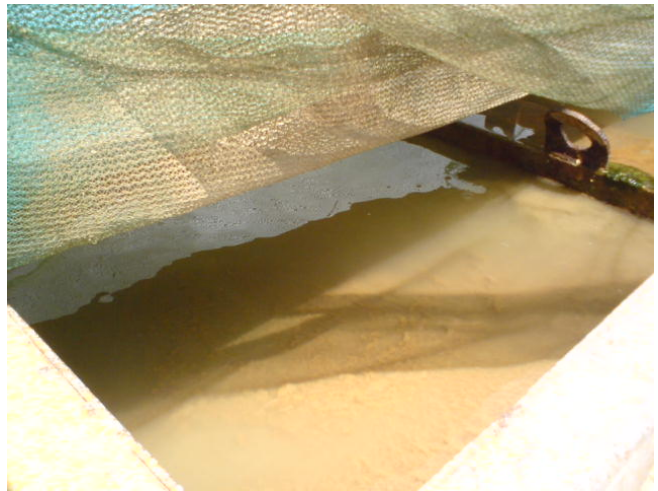
4. Cleaning of the de-slitting tank (Ko Po Road) should be performed to improve the efficiency of the tank.
