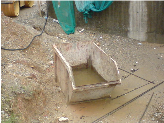
1. The stagnant accumulated in the lifting skip should be removed to prevent mosquitoes breeding
