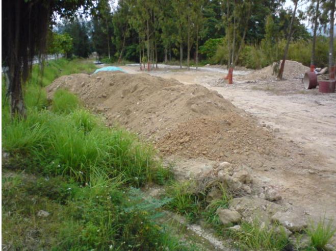
1. The soil stockpile in the site (Kam Tin River Ch.150-200) should be covered with tarpaulin sheet and the weeds accumulated in the U-Channel should be removed in order to prevent the blockage of the stream.
