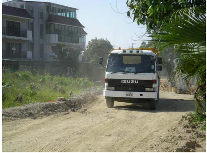
Dust control measures should be done to minimize the dust nuisance to surrounding residents.
