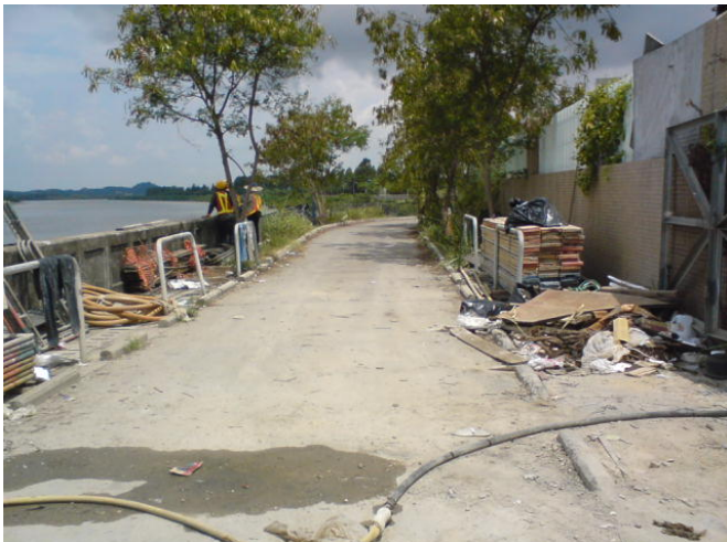
3. The contractor was reminded to maintain the site area clean and tidy. (Nam Sang Wai Pumping Station)
