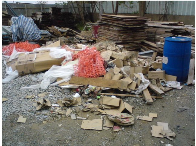
2. The C&D waste scattered on the site should be removed in order to maintain the site area clean and tidy.
