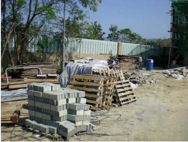
Entrance should keep clear and reminded to dispose waste properly.
