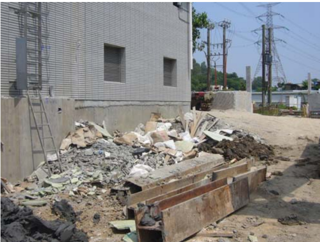
1. The C&D waste scattered on the site at Sha Po Pumping Station should be disposed properly in order to maintain the site area clean and tidy.
