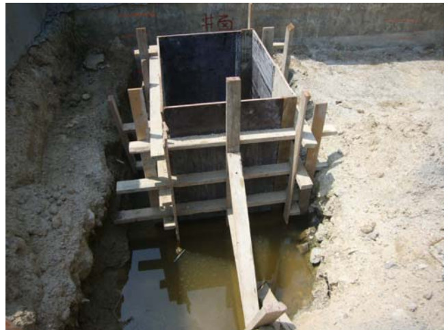
2. Stagnant water cumulated at Sha Po pumping Station should be cleaned to prevent mosquito breeding.
