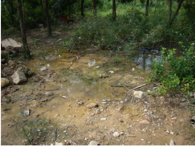
1. Stagnant water cumulated at Nam San Wai Road, the contractor was reminded to clean to prevent mosquito breeding.
