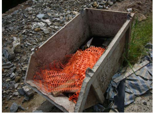
2. Stagnant water cumulated inside the waste skip, the contractor was reminded to clean ASAP.
