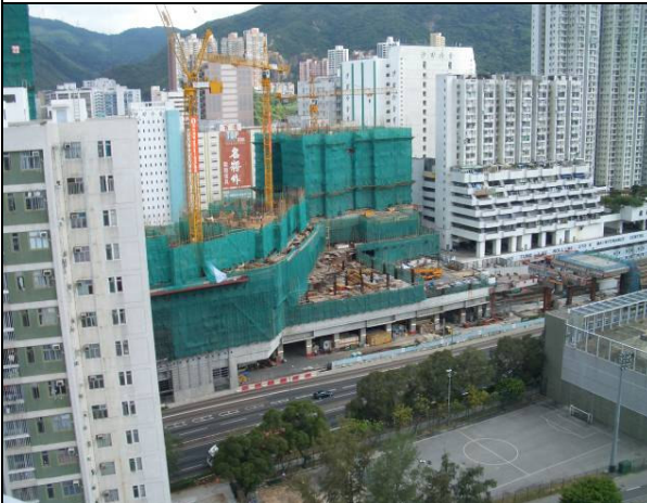
Photo 3: Construction works of the Ho Tung Lau project near NM1 and NM2.
