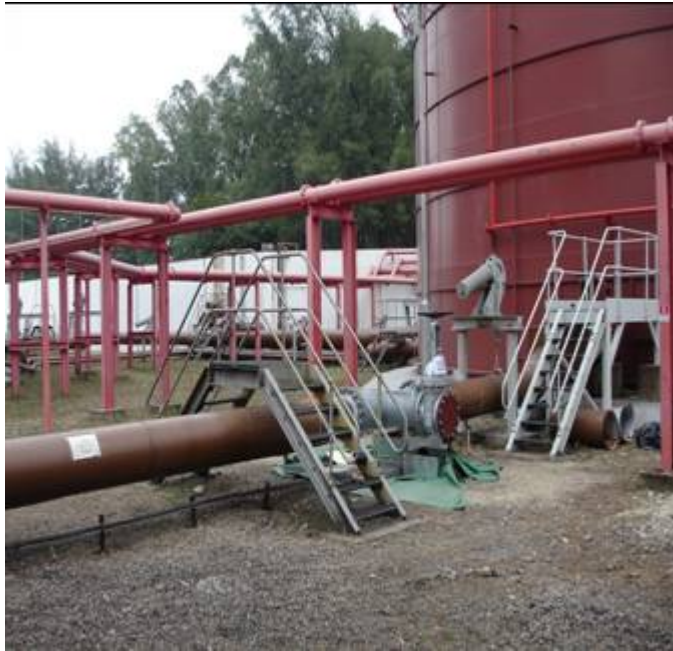
E.3 Fuel oil transfer line tie-in at CPA Fuel Oil Tank No. 2
