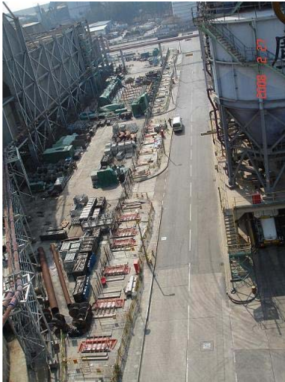
E.4 Construction of pipe support footing for relocation of underground pipe works
