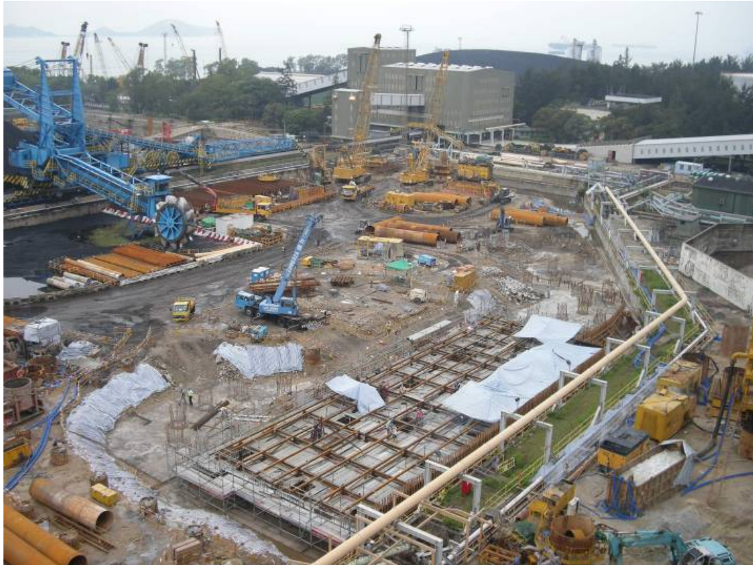
E. 1 Pile cap construction for the FGD Absorber of Units B1 and B2
