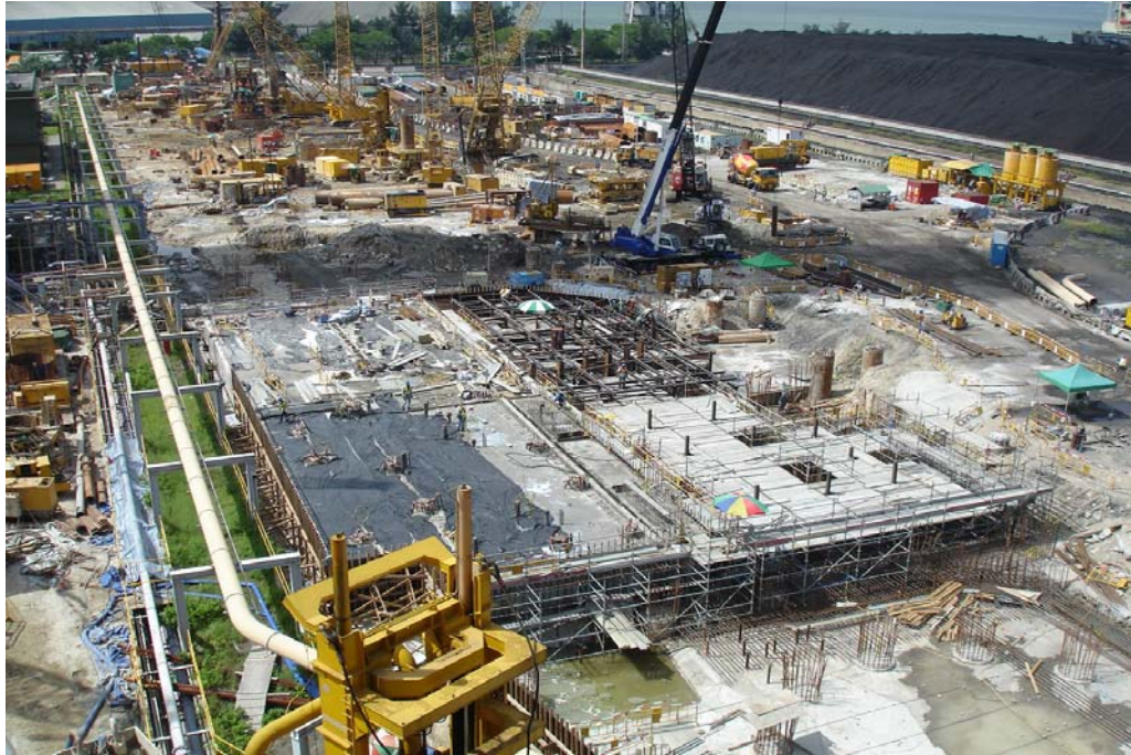
E. 1 Pile cap construction for the FGD Absorber of Units B1 and B2
