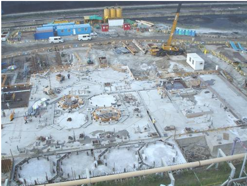
E.2 Pile cap construction for the common Limestone Preparation and Gypsum Dewatering areas
