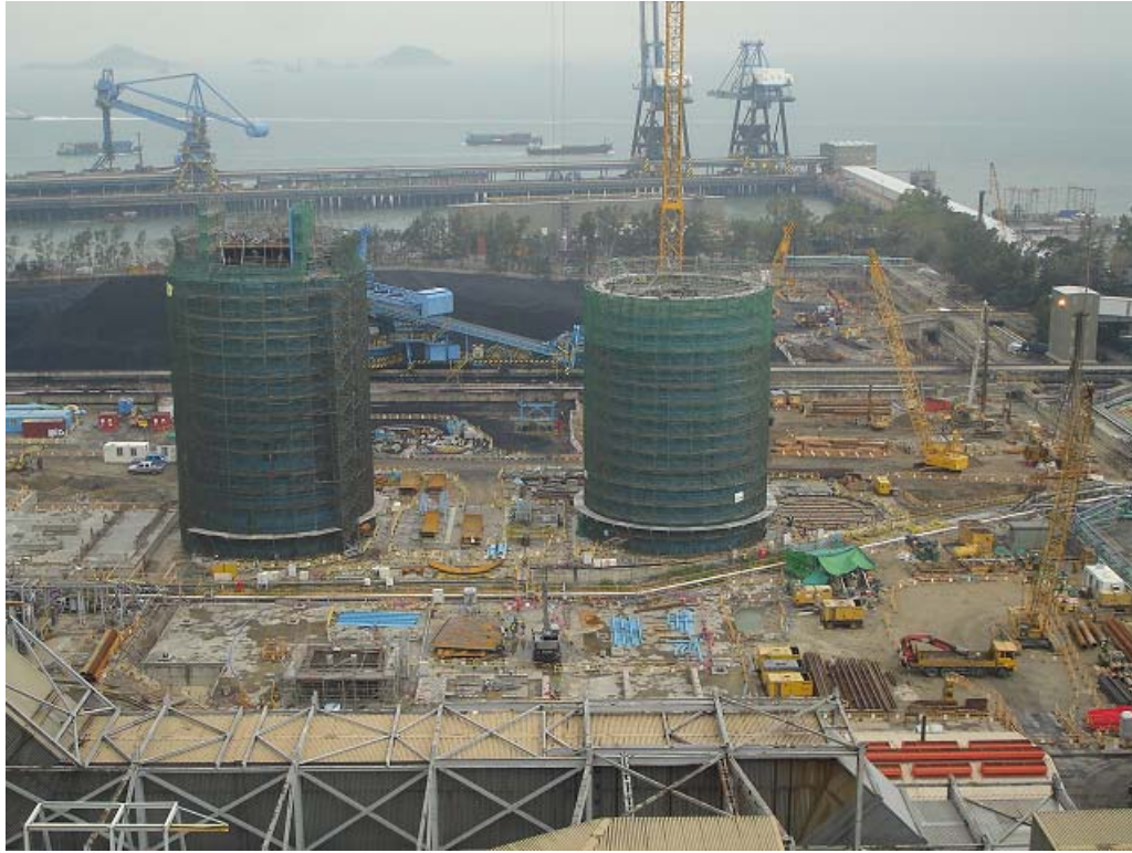
E. 1 Mechanical erection works of Unit B1 and Unit B2 FGD Absorbers
