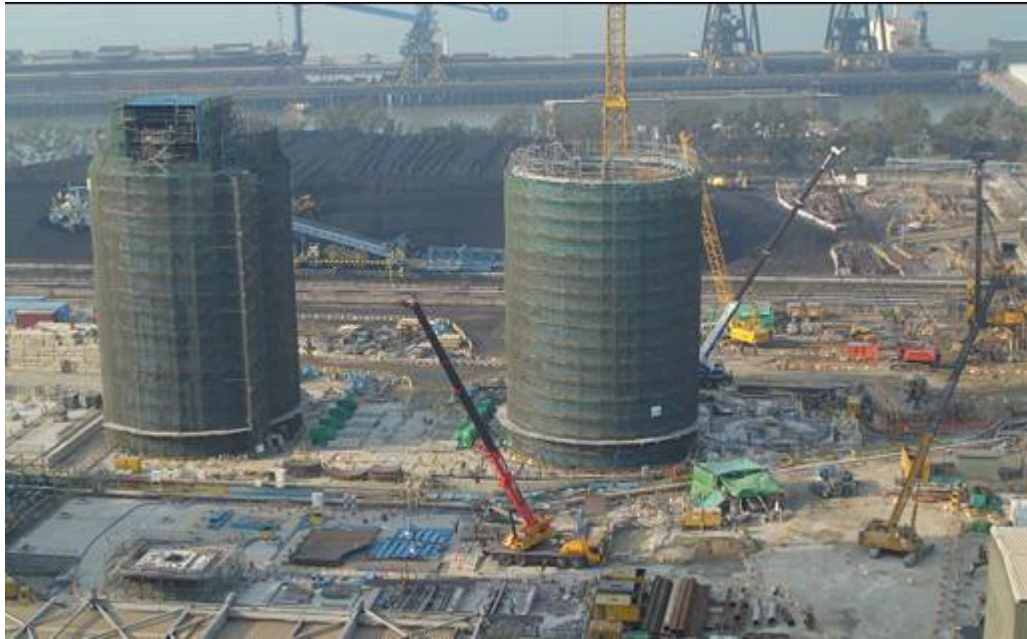
E.1 Mechanical erection works of Unit B1 and Unit B2 FGD Absorbers
