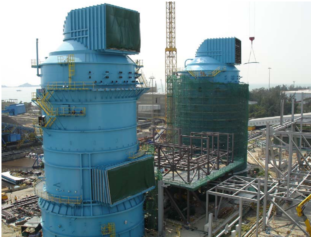
E.1 Unit B1 and Unit B2 FGD areas
