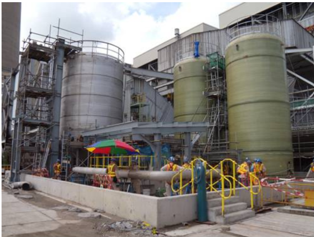
E.4 Urea Handling Area
