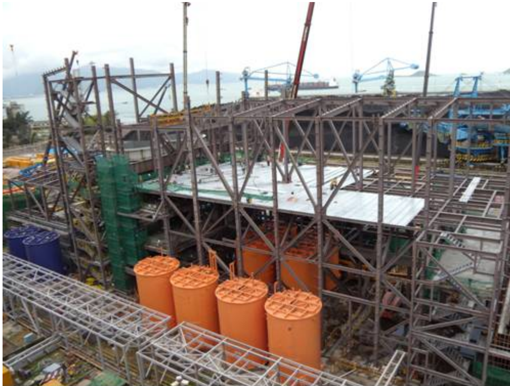
E. 2 Common Limestone Preparation and Gypsum Dewatering Areas
