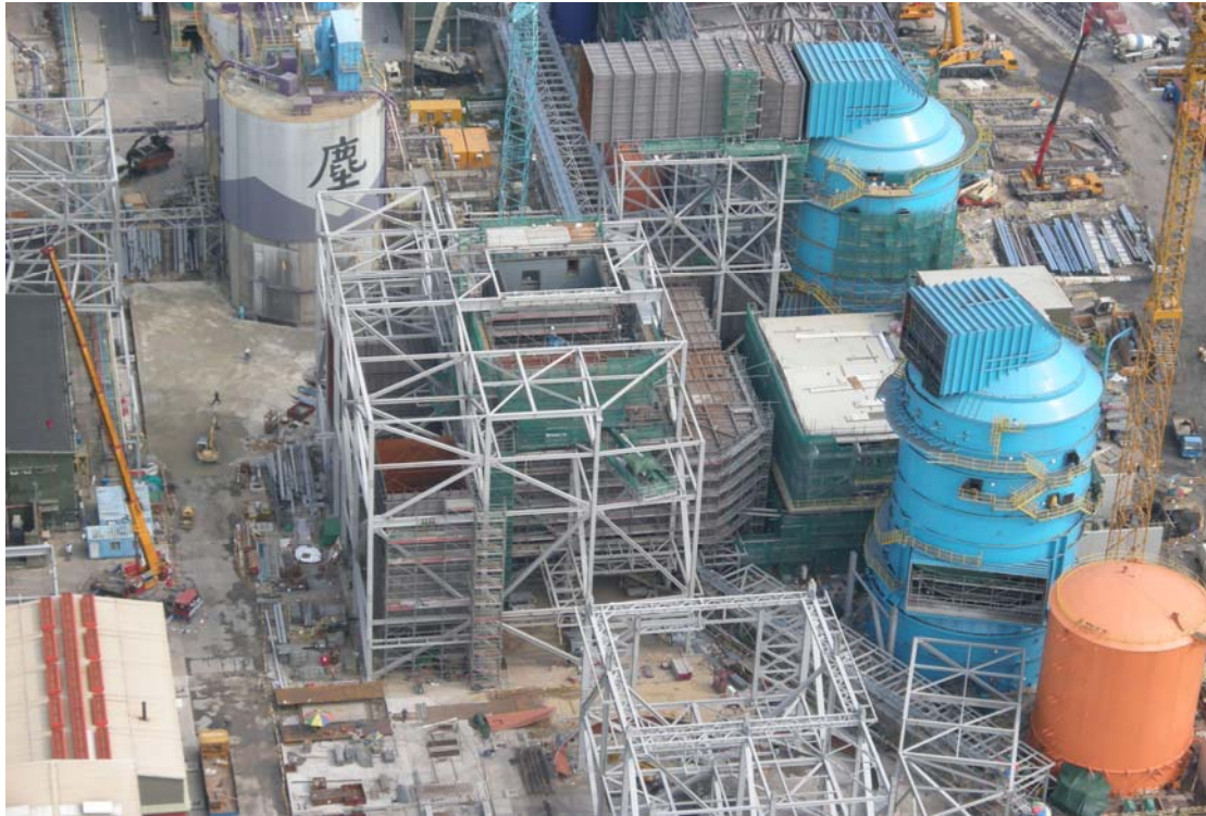
E. 1 Unit B1 and Unit B2 FGD Areas
