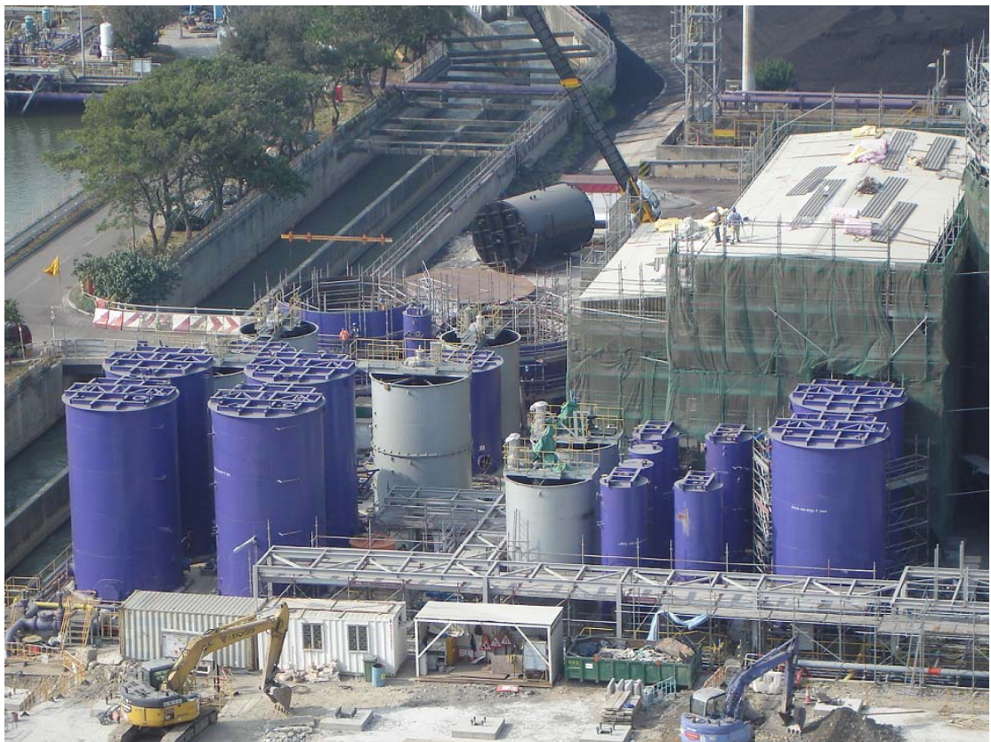
E.4 Waste Water Treatment Plant Area
