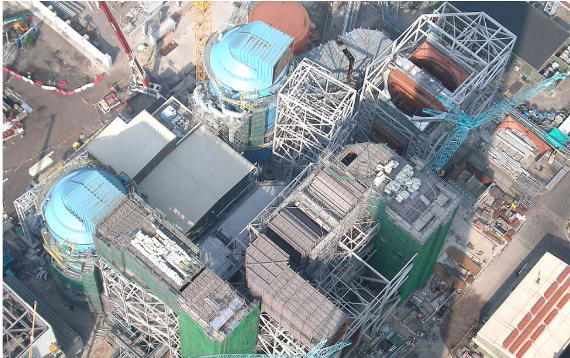
E. 1 Unit B1 and Unit B2 FGD Areas
