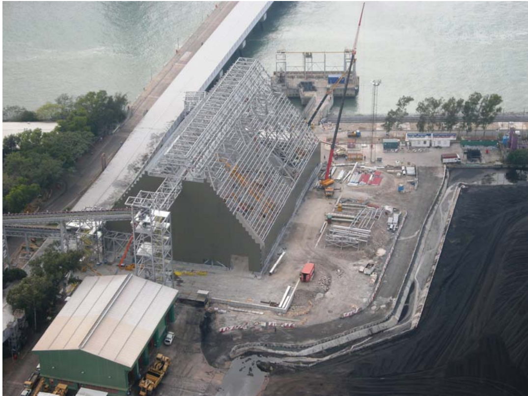
E.3 Gypsum Handling Area
