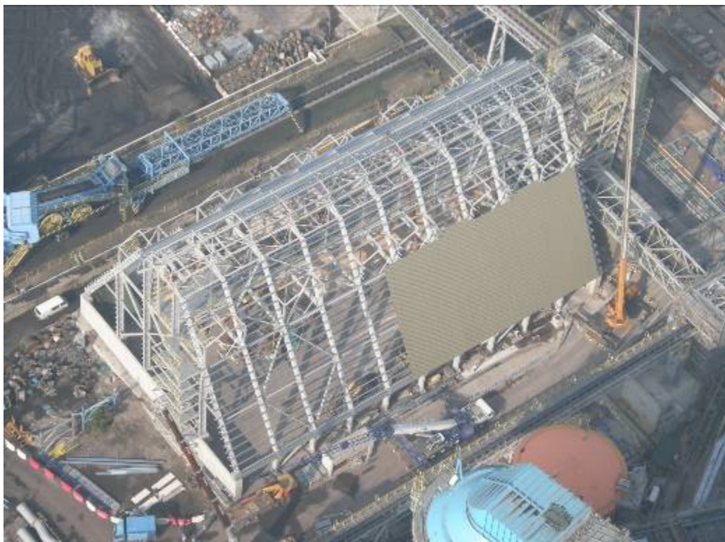
E.2 Limestone Handling Area
