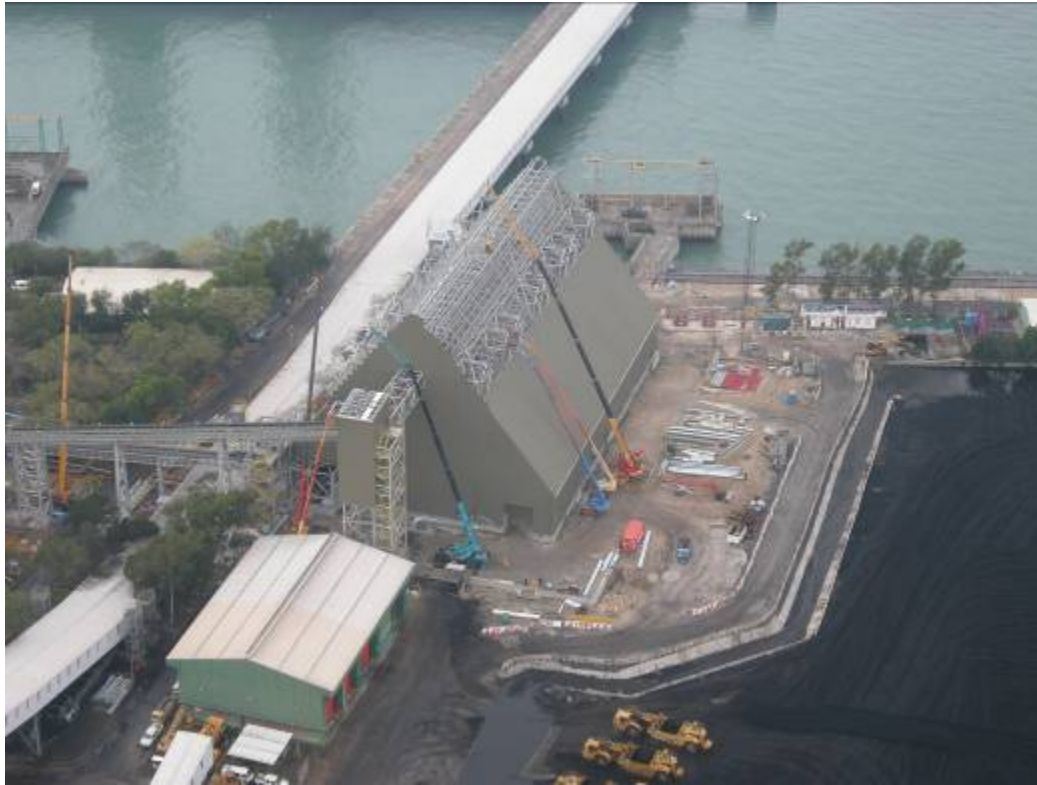
E.3 Gypsum Handling Area
