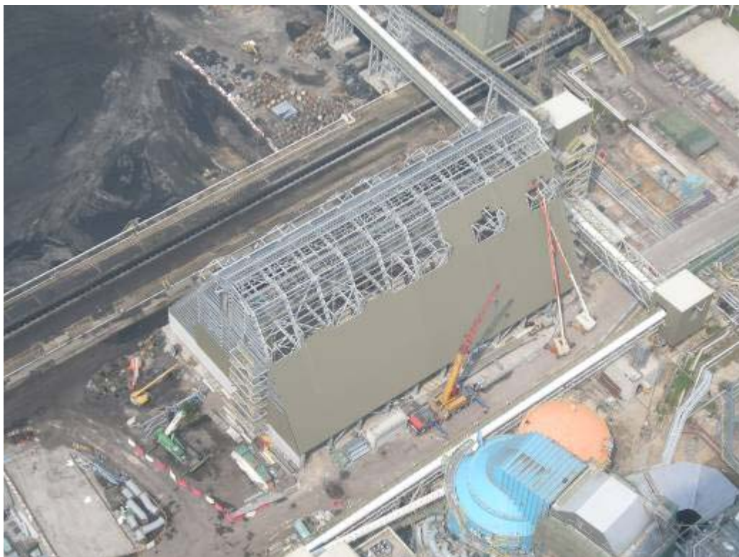
E.2 Limestone Handling Area
