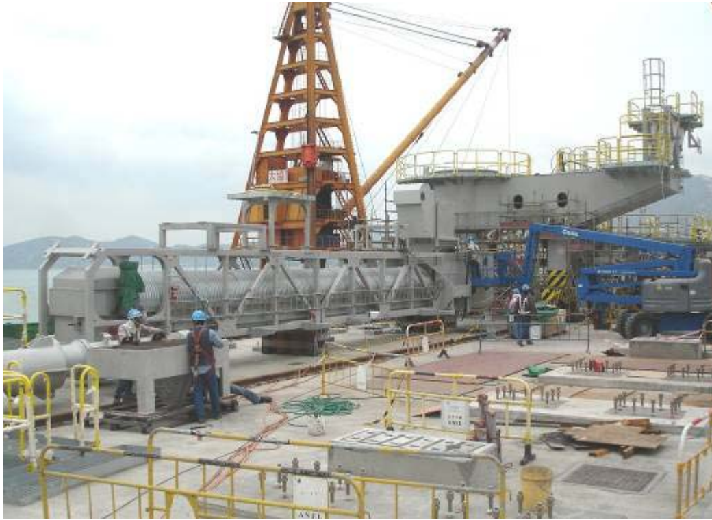
E.3 Loader/ Unloader at Material Handling Berth
