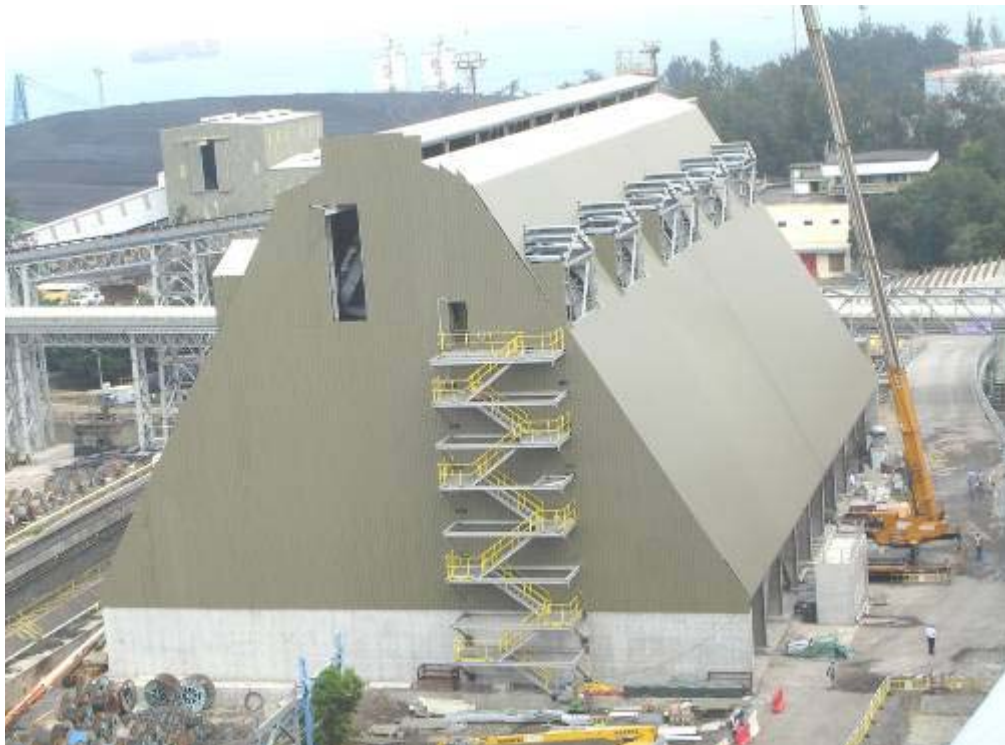
E.2 Limestone Handling Area
