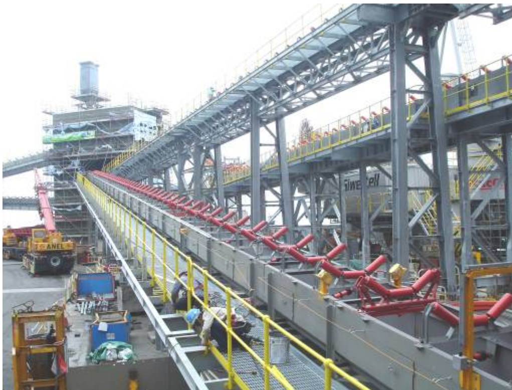
E.4 Material Handling Conveyor System at Material Handling Berth
