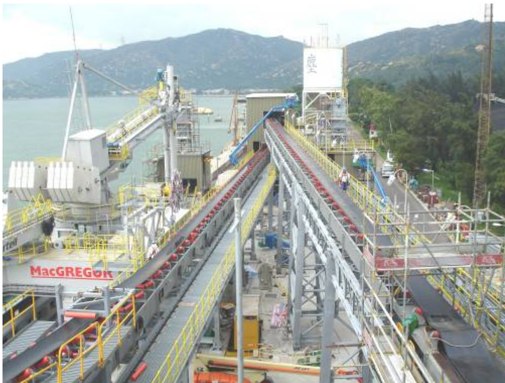
E.4 Material Handling Conveyor System at Material Handling Berth
