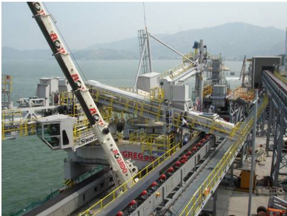
E.4 Loader/ Unloader at Material Handling Berth
