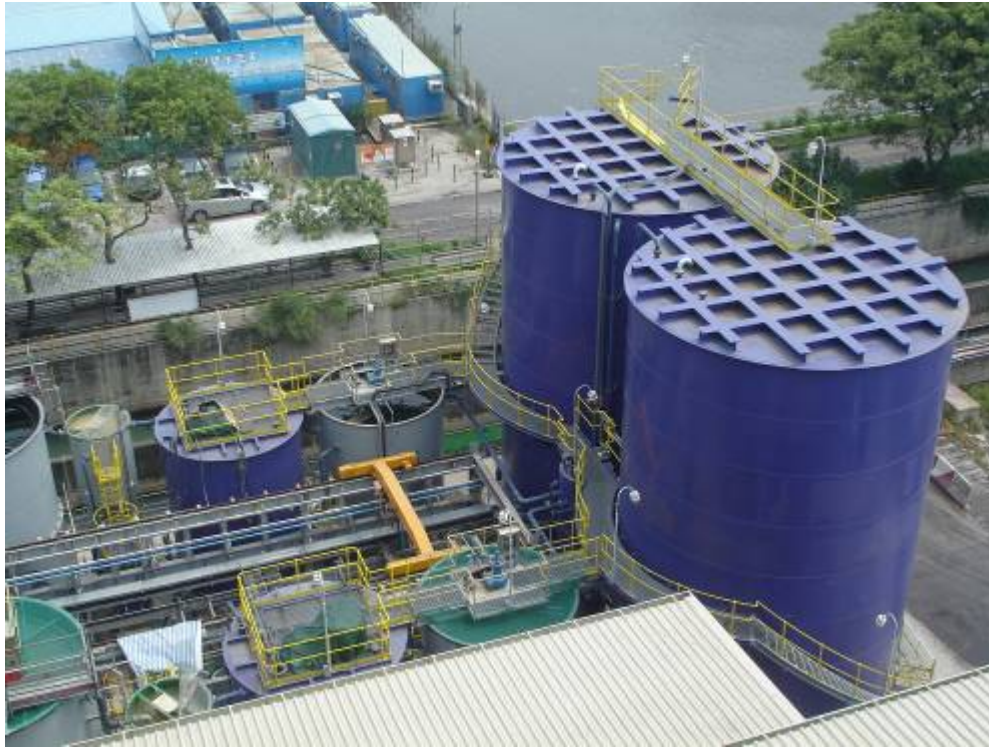
E.3 Waste Water Treatment Plant Area
