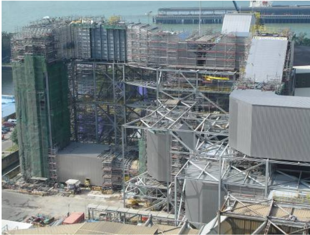
E.1 Unit B4 FGD Area
