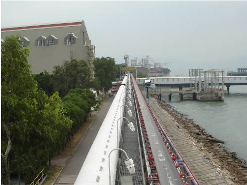
E.3 Material Handling Conveyor System
