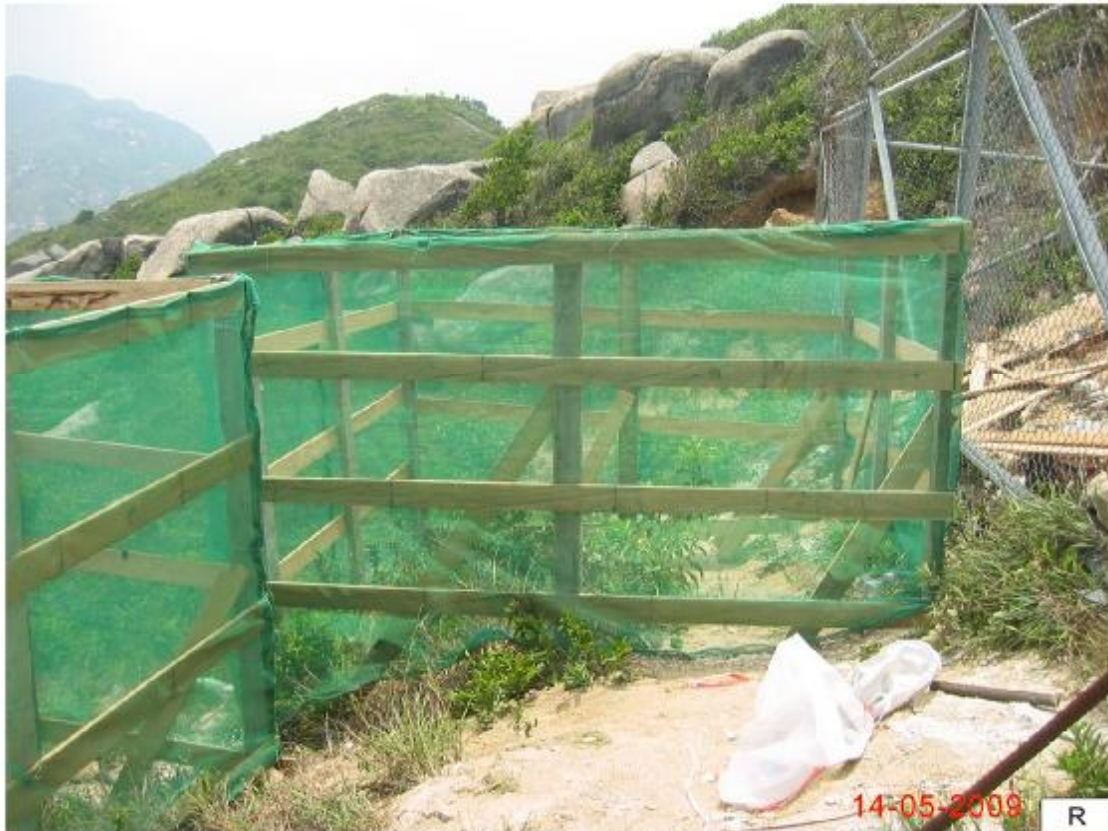
T5A with Plant Protection Fence
