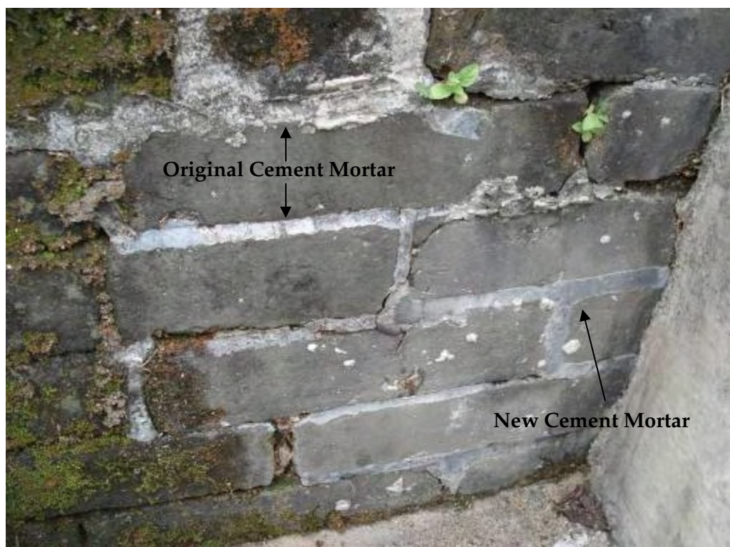
Figure 3.2g Comparison of original and new cement mortar of grave bricks (photo taken on 9 January 2010)
