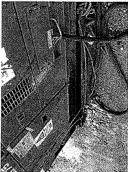
Photo 110817_001 (Standing Water was noted in drip trays after raining)
