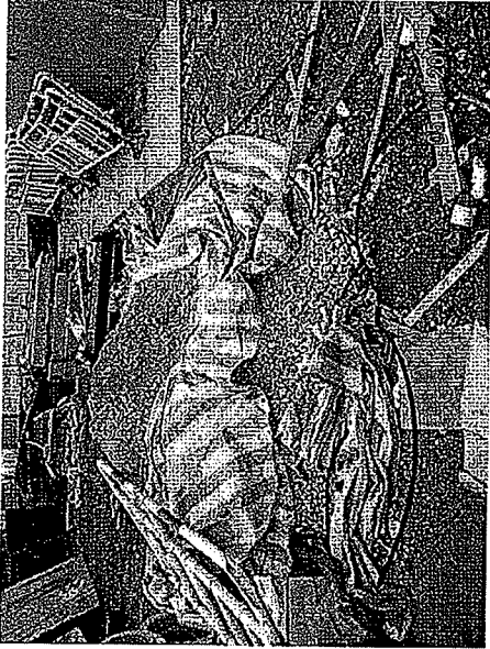
Photo_120105_002 (Some construction waste materials were noted in Portion J)
