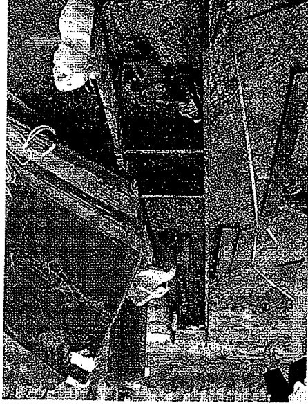
Photo_120117_002 (Standing water noted in Portion J were cleaned immediately)
