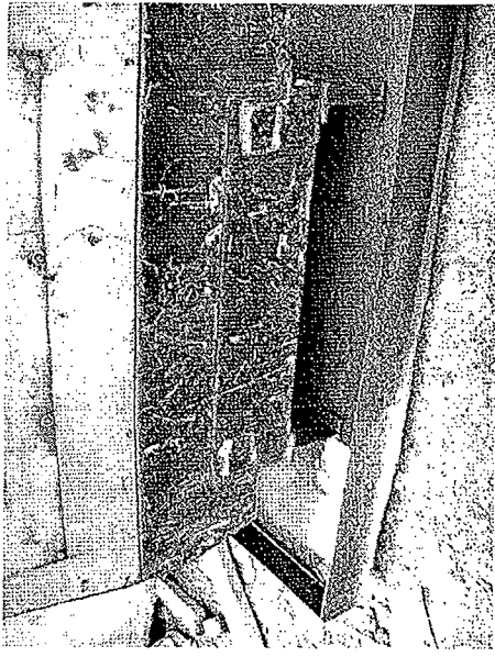
Photo_120612_003 (Standing water was noted in Portion J.)
