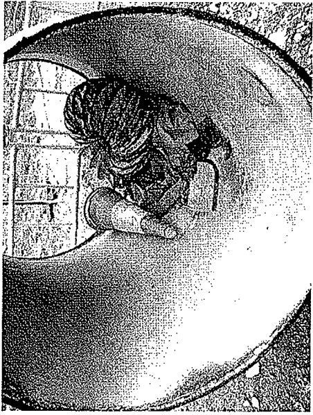
Photo_120612_001 (Standing water was noted in Portion H.)
