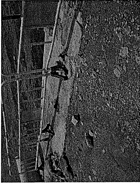
Photo_120718_001 (A gap was noted near the sea wall in Portion J.)
