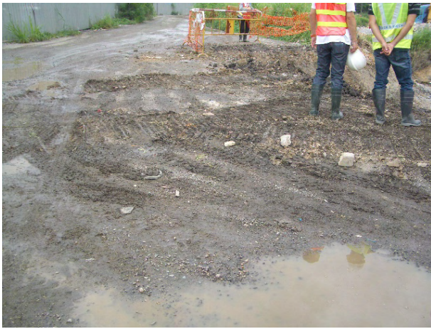
1. Stagnant water was cumulated at TKL-07 after the rain fall; the contractor was reminded to clean to prevent mosquito breeding.
