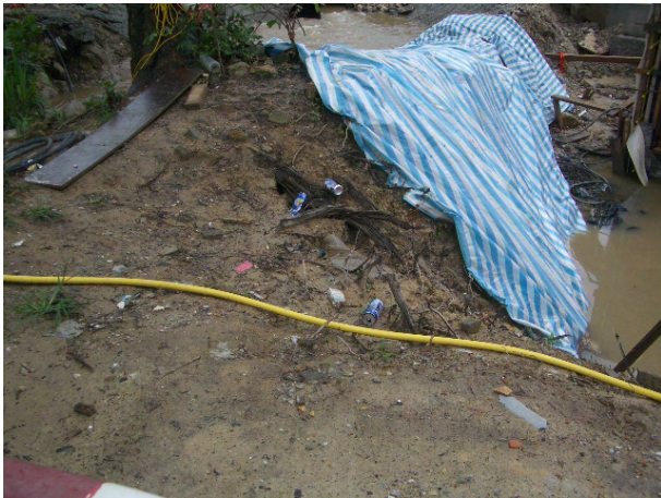
1. General waste scattered on site was observed at TKL-07, housekeeping should be improved to keep the site clean and tidy.
