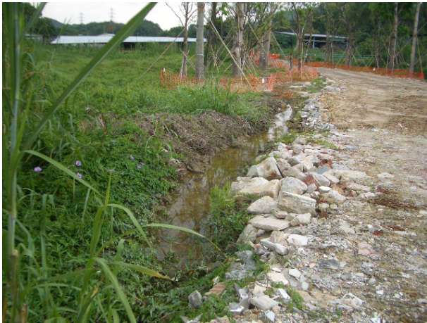
1. Stagnant water was cumulated at MUP; the contractor was reminded to clean to prevent mosquito breeding.
