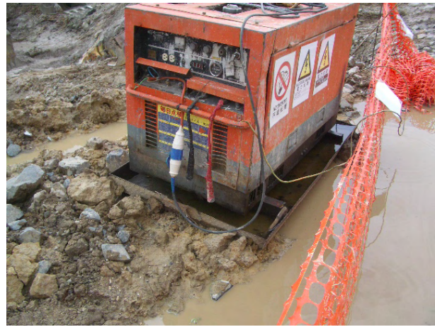
2. Stagnant water was cumulated inside the drip tray was observed at TKL-07; the contractor was reminded to clean to prevent mosquito breeding.
