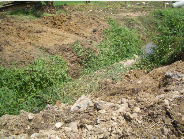
1. The C&D material should be removed from the channel at TKL02; the contractor is reminded to ensure all water channels without any blockage.
