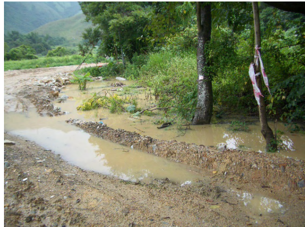
2. Stagnant water was cumulated at TKL-07; the contractor was reminded to clean to prevent mosquito breeding.
